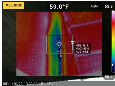
Figure 7: Consider Sealing the Seam in the Training Center IT Room Wall
