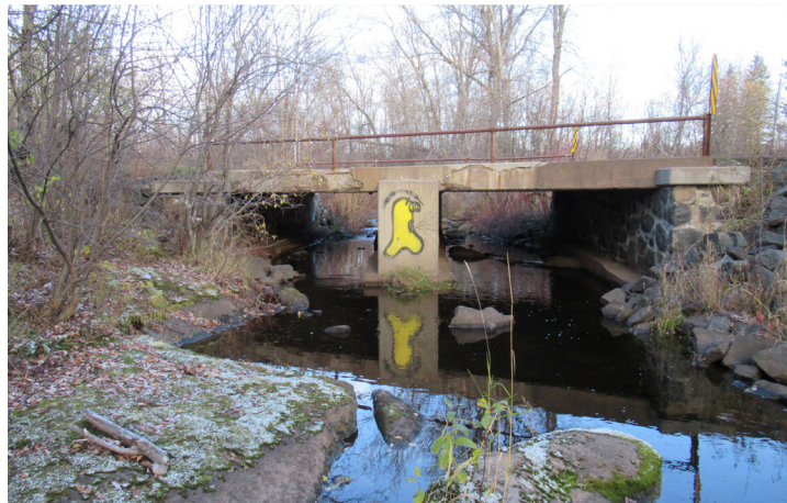
The existing two-span, in-place concrete slab bridge is founded directly on shallow bedrock.
