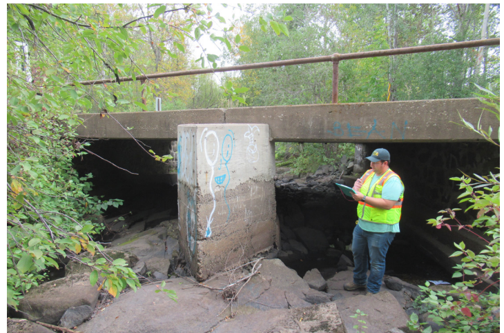
LHB conducted the bridge study report and is ready to start on the design.
