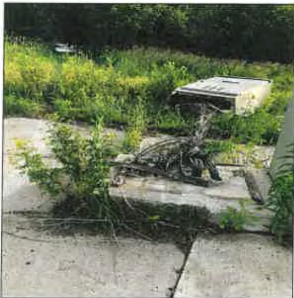
Electrical Damage Response Maple Grove Road
