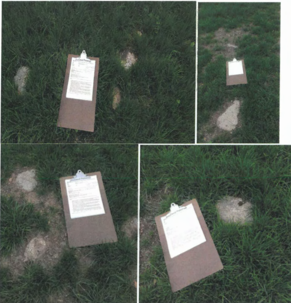
Photos: Noted large debris and unestablished grass in topsoil at northeast area of building/site.
