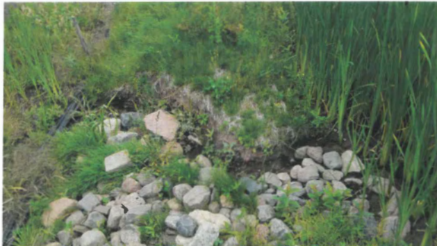
Photo: East side of pond; erosion at riprap.
